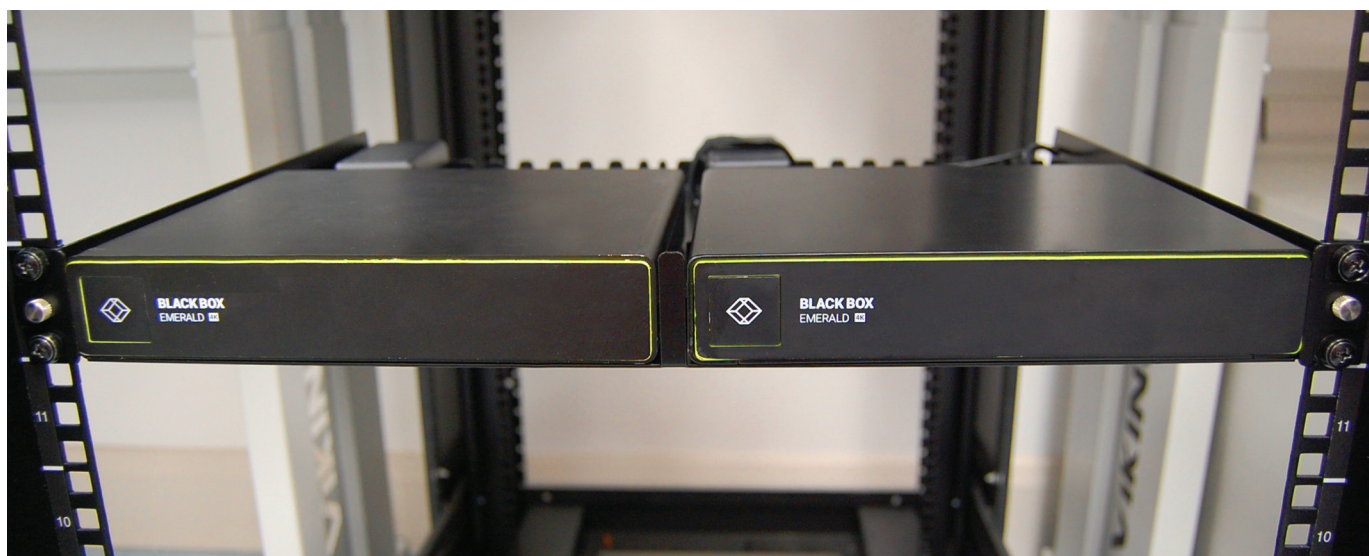
FIGURE 2-5. TRANSMITTERS OR RECEIVERS INSTALLED
